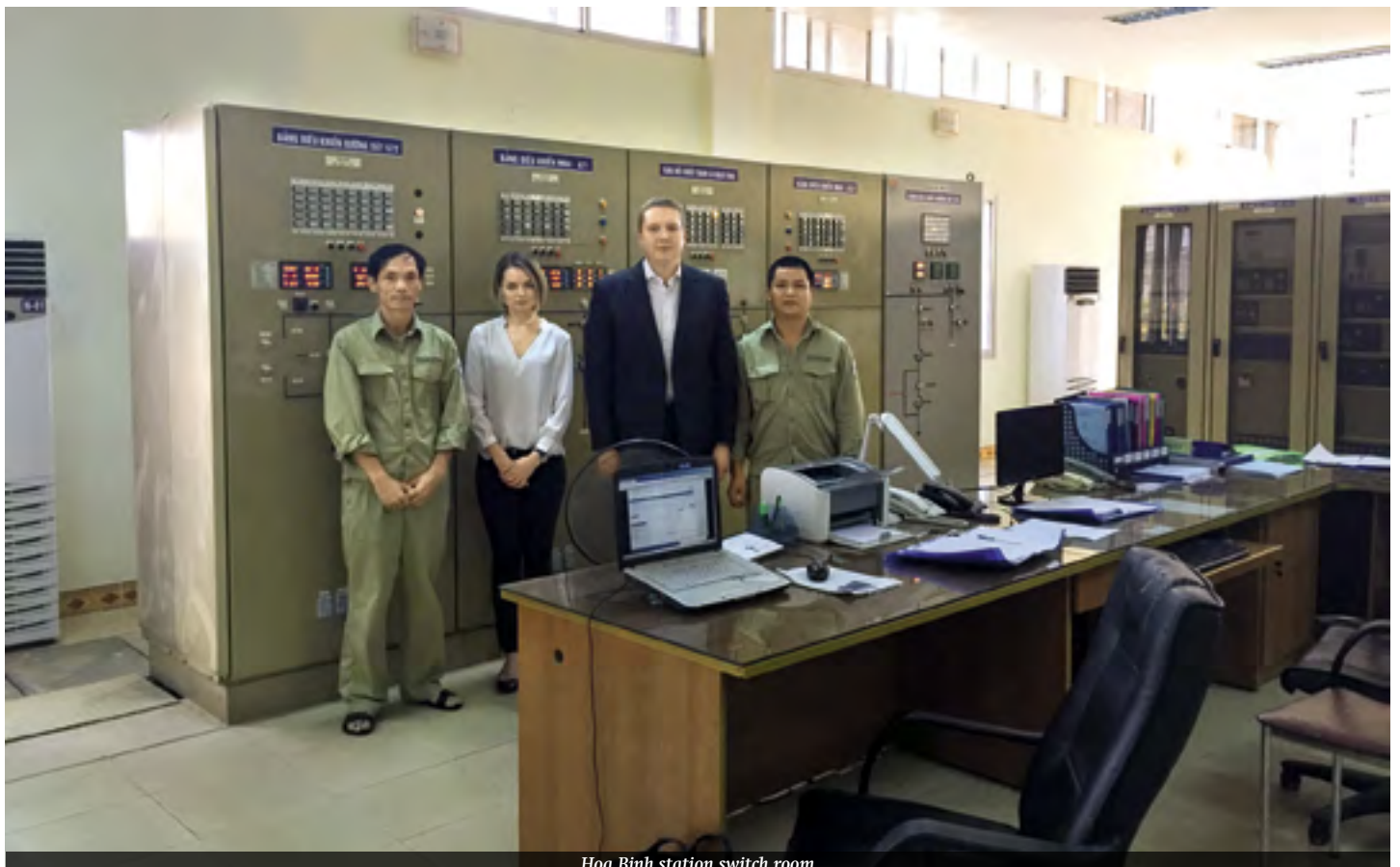
Hoa Binh station switch room
