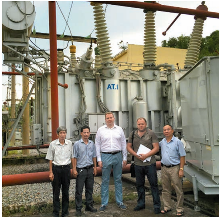
Hoa Binh HPC. HV bushings have served for over 30 years proving the high quality and longevity of Izolyator products
