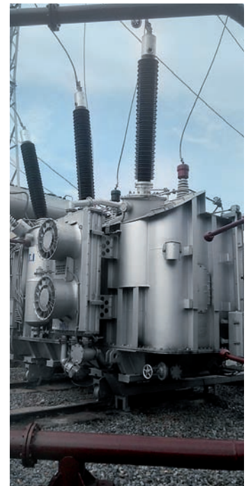
220 kV RIP bushings installed in transformers at Hoa Binh HPC in 2016
