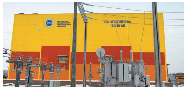
Substation Polyanka in Moscow Region. Photo from official website of MOESK
