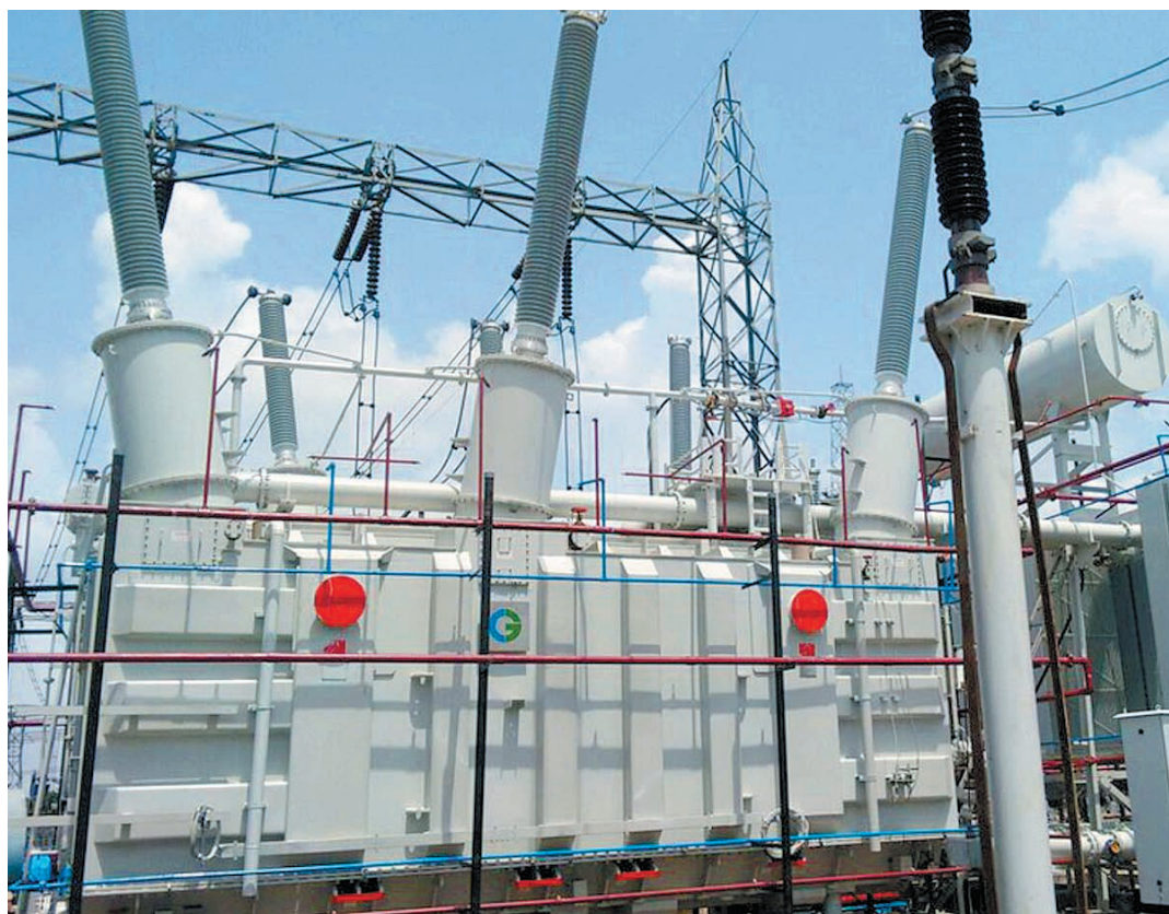
Izolyator bushings in a transformer at Bamnauli substation
