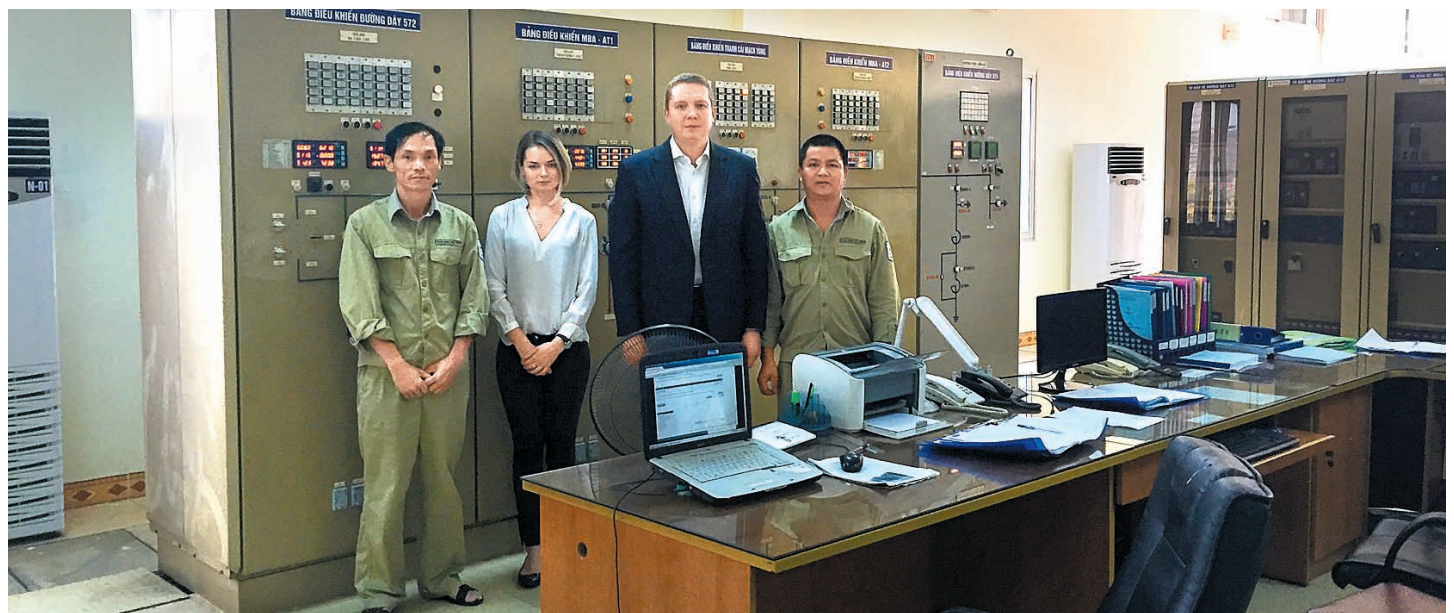
In the switch room of Hoa Binh HPP. April 2015
