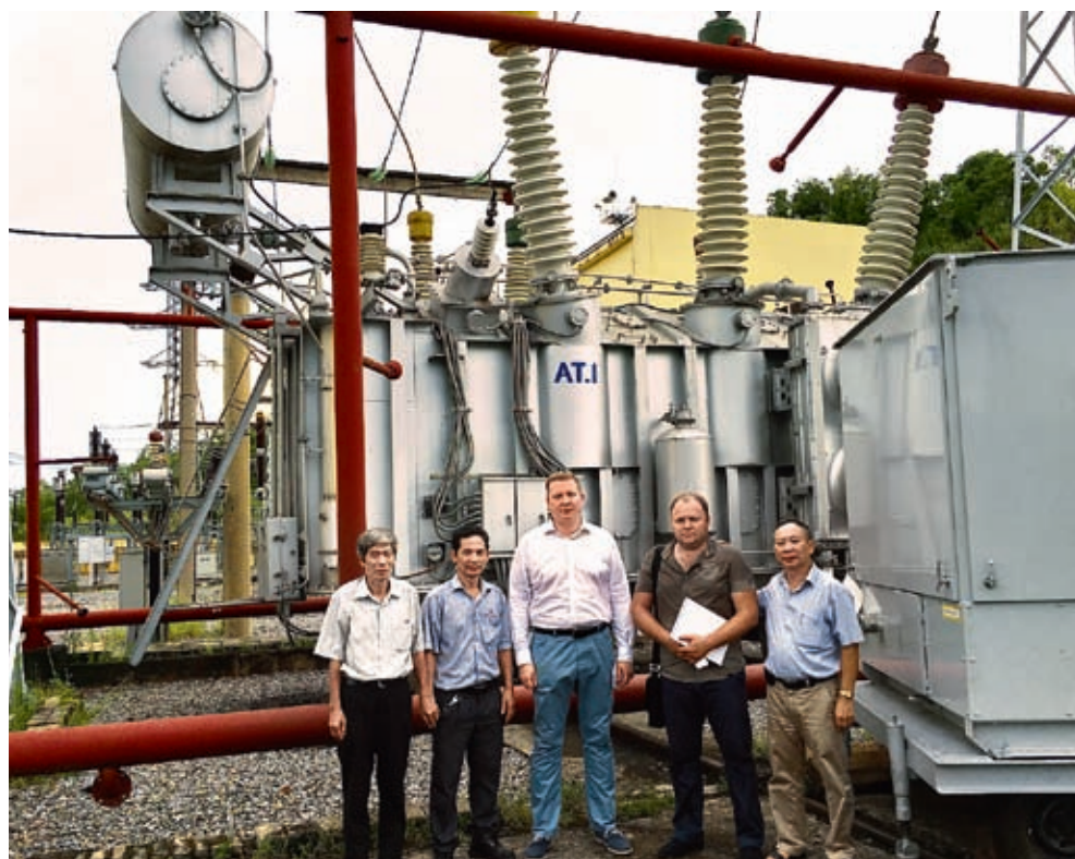
Participants of the meeting at Hoa Binh HPC. In the background: transformer with Izolyator bushings, 30 years in operation
