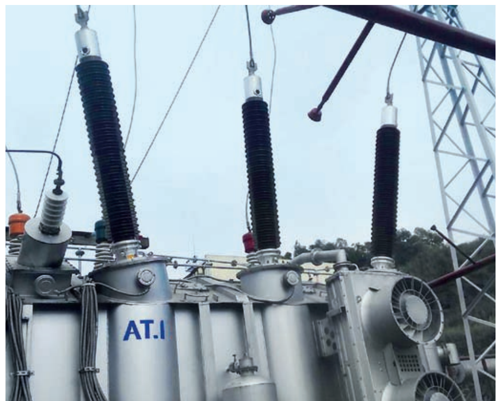
220 kV RIP bushings delivered by Izolyator to Hoa Binh in 2016
