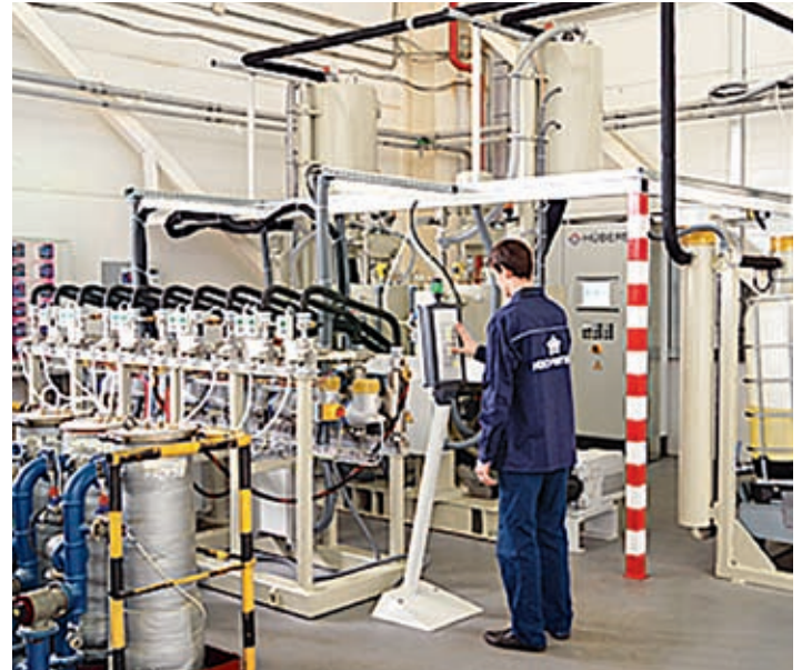
Airvoid mixing and dosing Hübers unit at Izolyator plant
