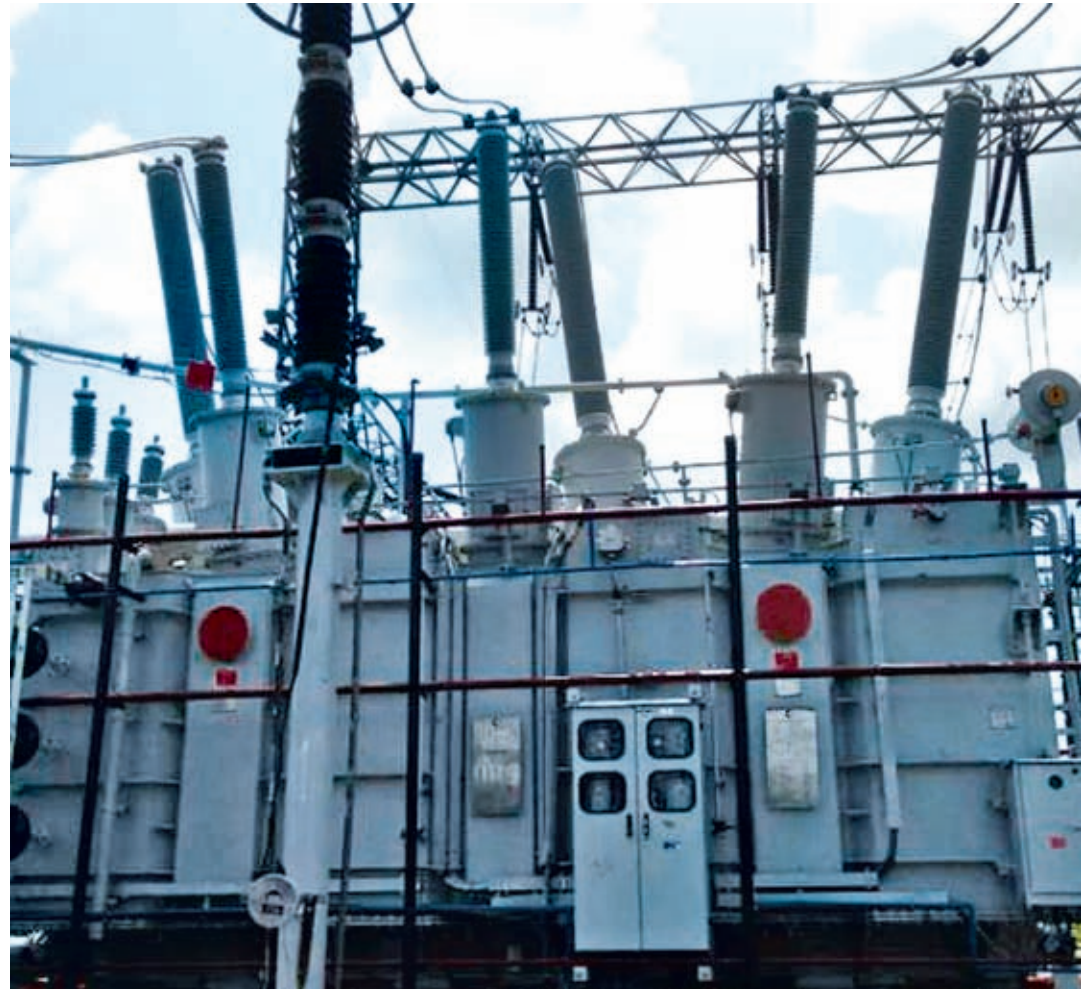
Transformer with Izolyator bushings at 400 kV Bamnauli Substation in India
