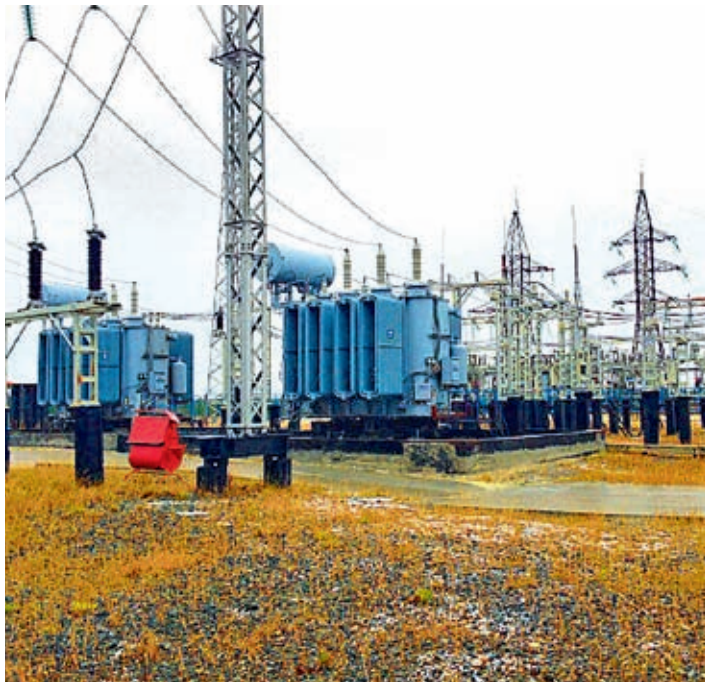
Package transformer substation (photo from official website of Electroshield Samara company)
