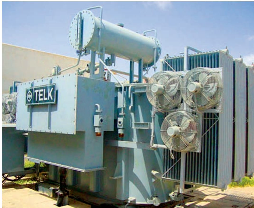
Photo from the official webpage of Transformers and Electricals Kerala Limited
