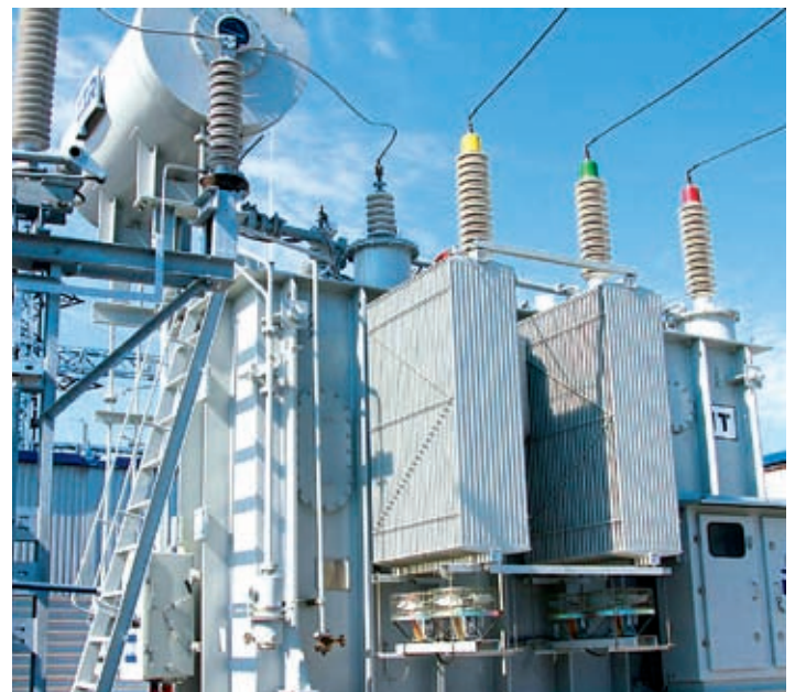
Transformer at Kuznechevskaya SS of Arkhenergo (photo from official webpage of IDGC North West)
