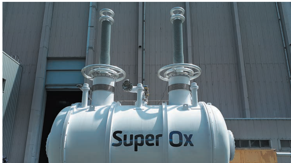
The first phase of the 220 kV superconductive current limiter, equipped with Izolyator bushings, at KERI test center
