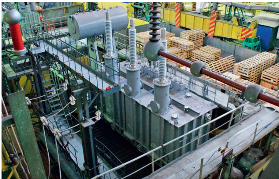
Compensating reactor with a 100 MVA capacity equipped with 220 kV Izolyator high-voltage bushings at the test field of the Togliatti transformer plant (photo: Togliatti transformer)
