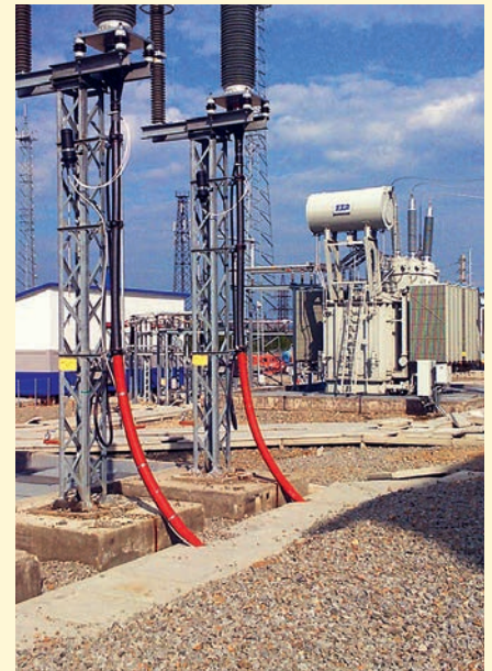
Transformers with Izolyator HV RIP bushings at the 220 kV Mogocha substation of the Main Power Systems of Siberia
