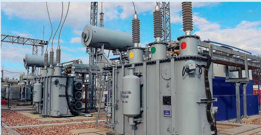
Transformers with Izolyator HV bushings in the 110 kV Ayanskaya substation in the Simferopol vicinity (photo: SUE RC Krymenergo)
