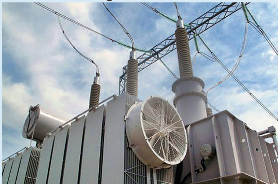
A 200 MVA autotransformer, equipped with Izolyator bushings at the 220 kV Severnaya substation in the Tula Region (photo: Rosseti FGC UES)
