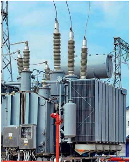
Transformers with Izolyator bushings at a 220 kV substation of MPS South (photo: Rosseti FGC UES)
