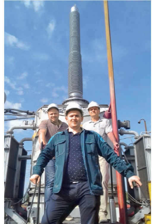
Installation done. L-R: Dmitry Mashinistov, Lead Engineer at Riko representative office in Belarus Anatoly Tereschuk and Chief of 750 kV Belorusskaya SS Vyacheslav Maskalik
