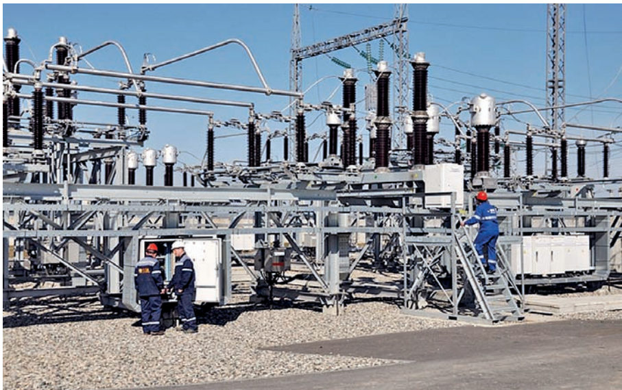
One of substations of Stavropolenergo (photo: Rosseti PJSC)
