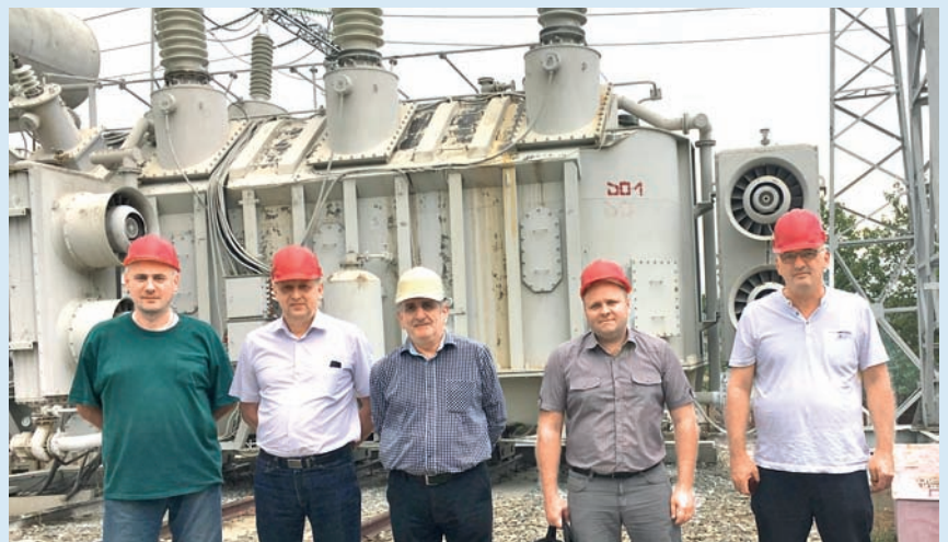
Workshop participants, L-R: Substation Chief Davit Chkheidze, Konstantin Sipilkin, Head of Transformer Repair Service of GSE Nodar Gavasheli, Dmitry Mashinistov and Aetos Ltd's Director Tamaz Sharikadze
