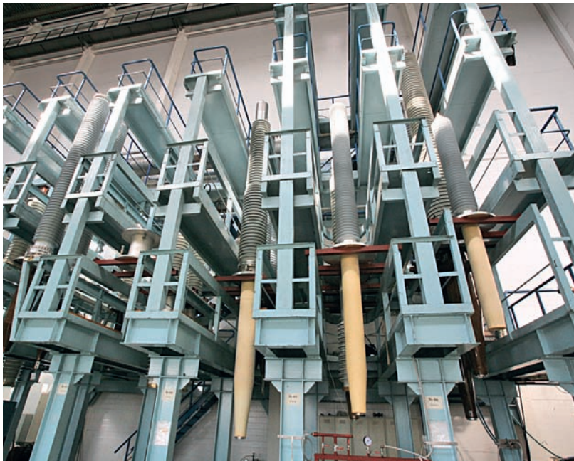
RIN bushings at the assembly shop of Izolyator plant
