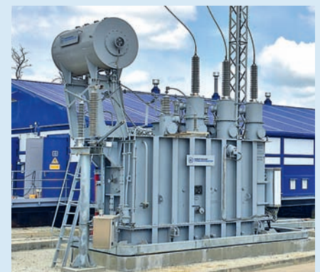
110 kV Aeroport substation (photo courtesy SUE RC Krymenergo)
