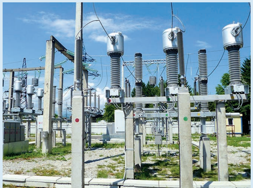
A Kabbalkenergo substation (photo courtesy RusCable media holding)
